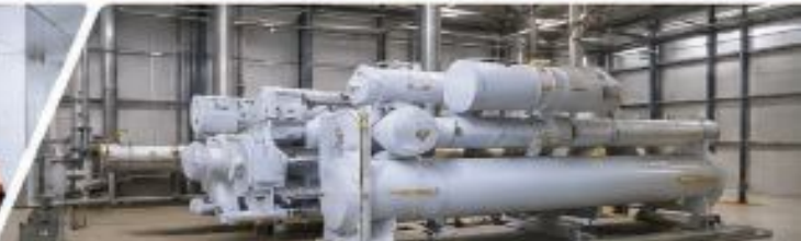
INDUSTRIAL REFRIGERATION SYSTEMS
